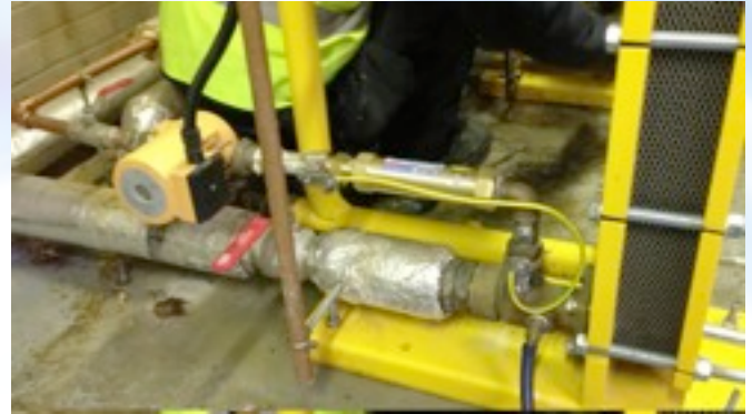
JFK Plumbing & Heating Ltd installed the patented AQUABION® water treatment systems
