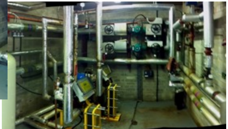
The Plate Heat Exchangers were under a constant costly repair program with a regular 6 monthly descaling program.
